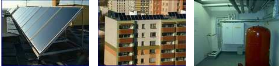
IMAGE 2 Solar panels for preparation of HW, reconstructed building, heat reservoir for solar panels
